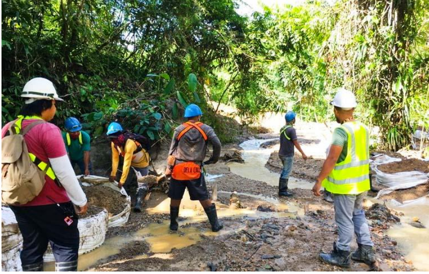
3 TVIRD Environment personnel conduct desilting activities after several days of constant raining.
